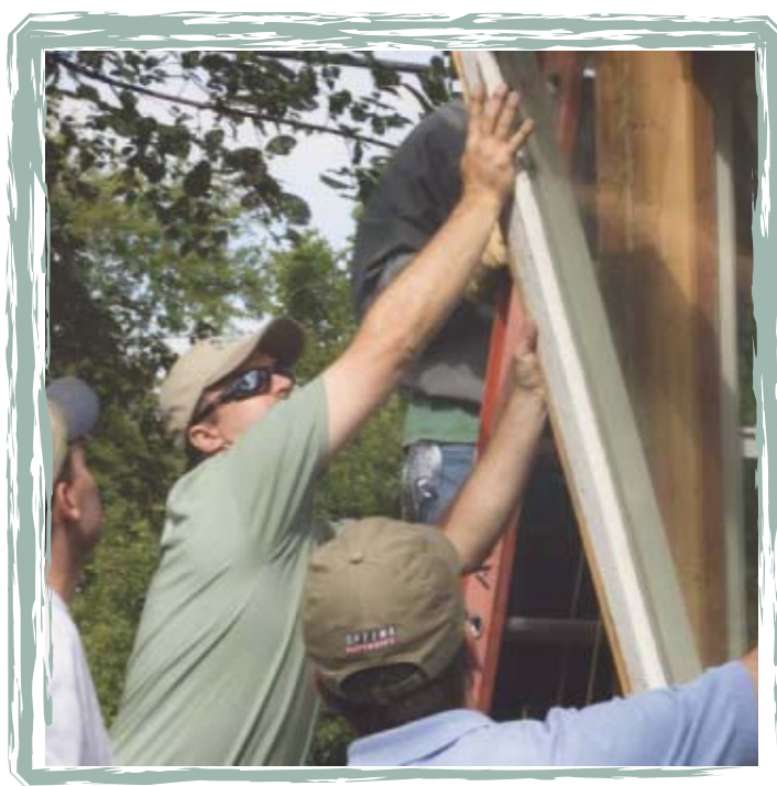
The Power of People. Volunteers from Rebuilding Together's Billings, Montana, affiliate tear down Jody Becker's old broken and rotting windows, floorboards and siding and install new, energy efficient components.
